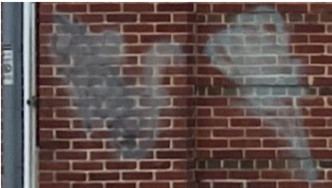
Before photo of graffiti on Chestnut Street.
