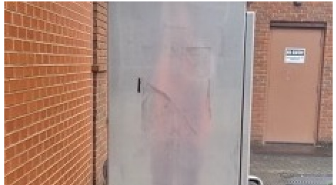
Graffiti removed off Chestnut St utility box.
