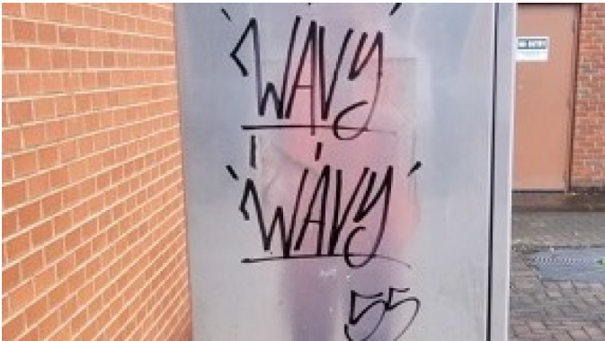
Graffiti on Chestnut St utility box.
