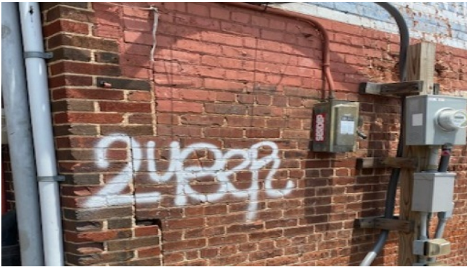
Graffiti on a building before cleaning.
