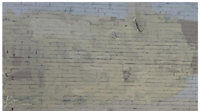
Graffiti painted over on 6th St.
