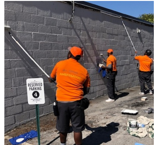
Ambassadors paint over a large graffiti tag on the back side of a district building.
