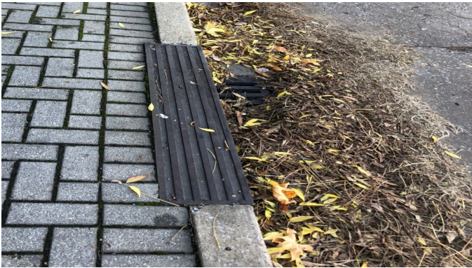
Catch basin 4th street before photo.
