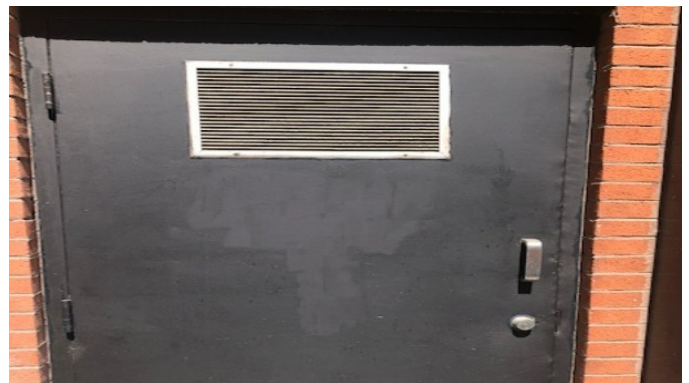
Graffiti removed from a door.
