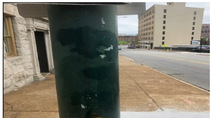
Graffiti removed from light pole.
