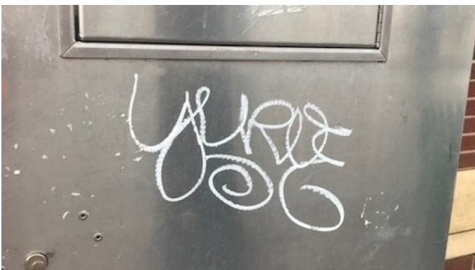
Graffiti on electrical box.
