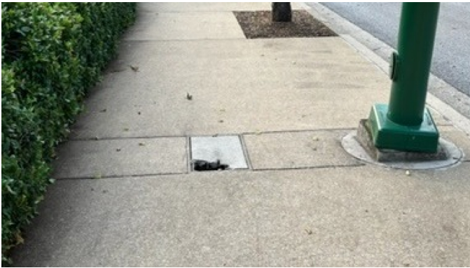
Sidewalk cover broken 3rd St.
