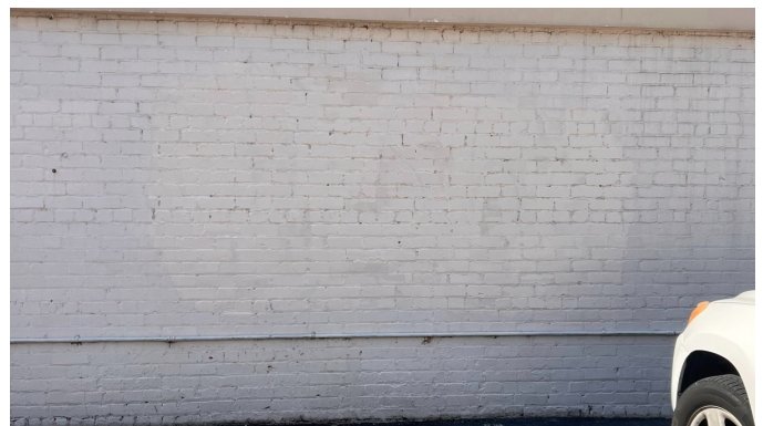
After photo of graffiti removed from Broad St.
