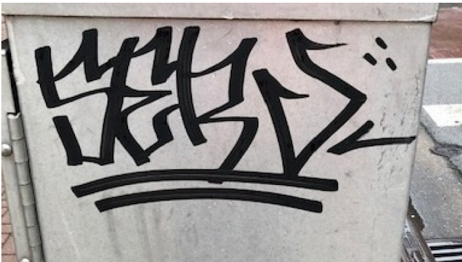
Graffiti on electrical box.
