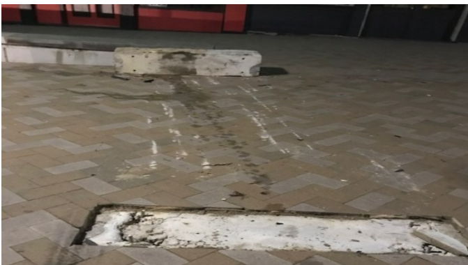
Parking block damaged by car.
