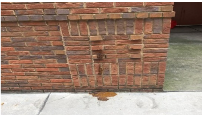
Biohazard before cleaning on 3rd St.
