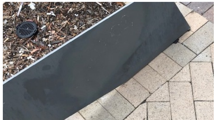
Graffiti removed from tree well on Patten Parkway.
