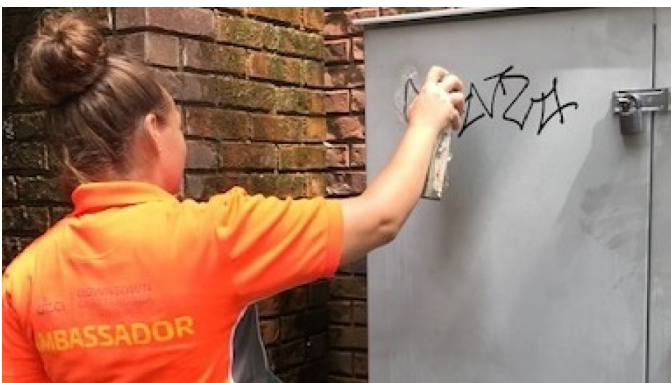
Graffiti on electrical box Chestnut St.
