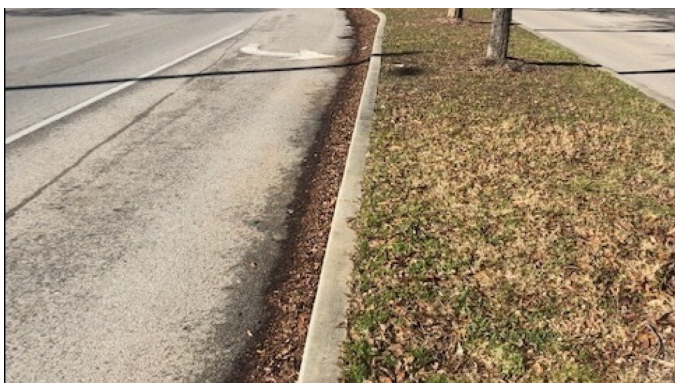
4th street center island before debris removed.
