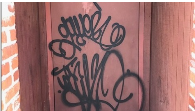
Before photo of Graffiti on 3rd St.
