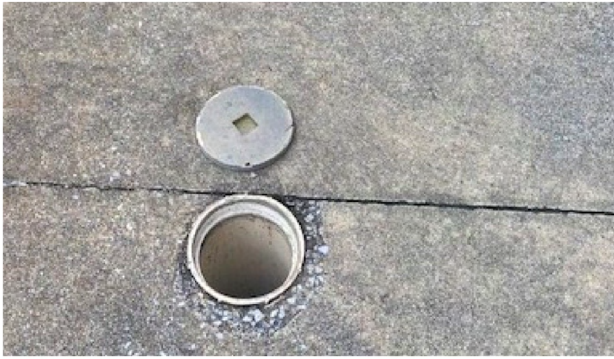
A cover came off the sidewalk on Broad St.
