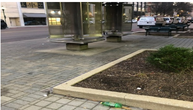
Debris at 8th and Market St.
