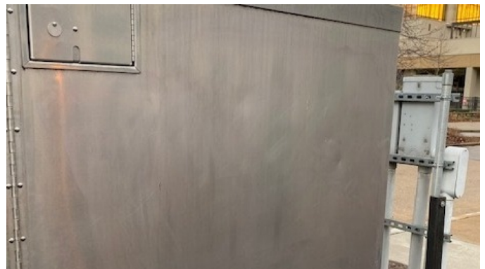
Graffiti removed off electrical box at MLK & Pine St.
