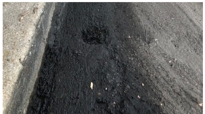
Debris removed from curb line.
