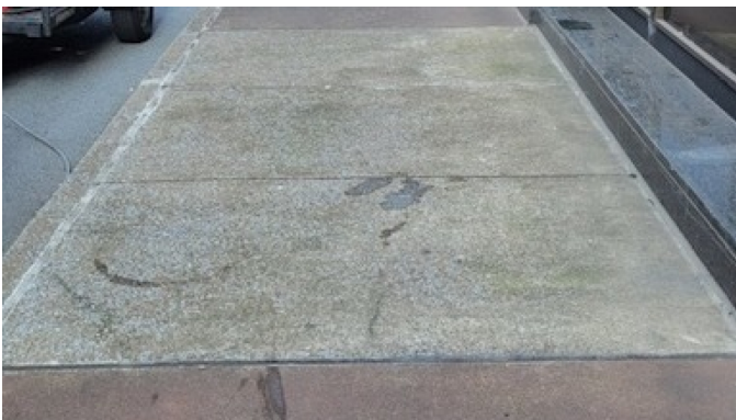
Sidewalk before power washing on 7th.
