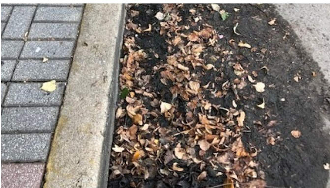
Debris in curb line.
