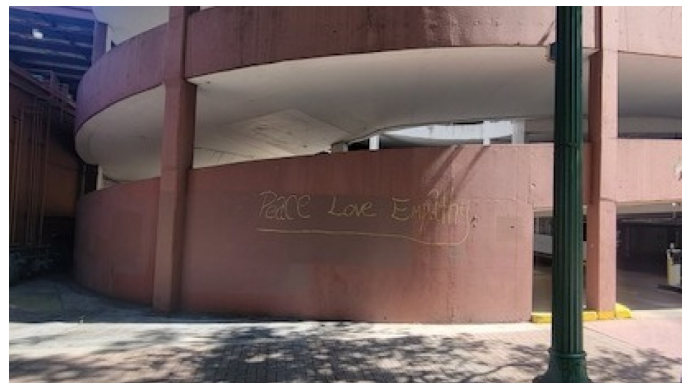
Chalk on wall Broad street building.
